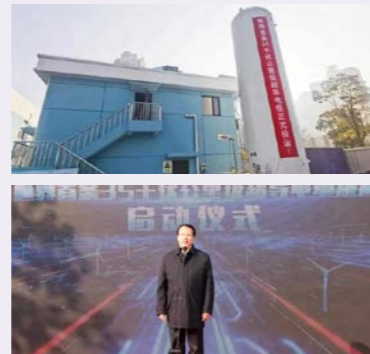
The world's first demonstration project of 35kV km superconducting cable designed by the Company was officially put into operation
