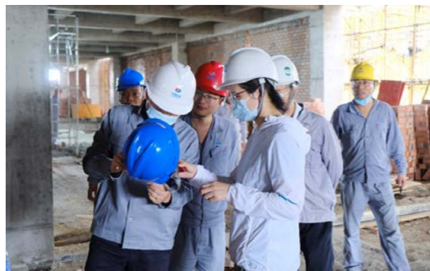
The Company's leaders led the team to inspect the general contracting project
