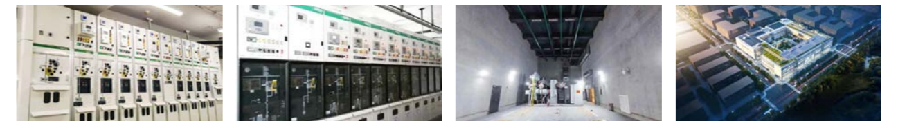
The first target distribution network double-loop network frame project in Xiong'an New District designed by the Company was put into operation
