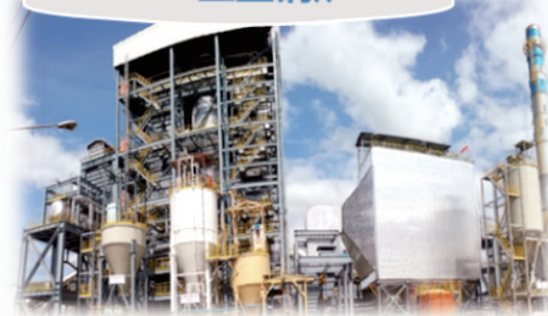
CFB工业锅炉
