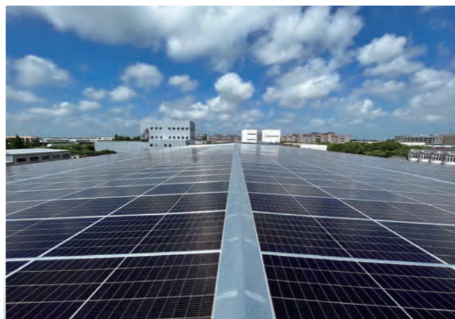
紫丹印务886KW-EPC光伏项目 Zidan Printing's 886KW-EPC Photovoltaic Project
